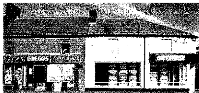
Corporate brand signs with lettering that completely disregards the location within a conservation area.
