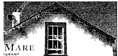
Floodlighting tucked under bargeboards achieves the objective of lighting the elevation, without the light fittings themselves being conspicuous.
