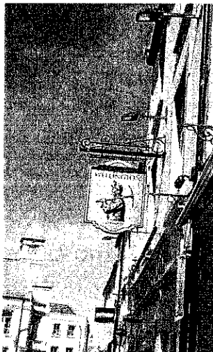
Projecting light fittings above first floor windows, further light fittings at fascia level and strip lights either side of the projecting sign.
