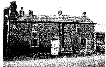
The appearance of this traditional building has been spoiled by the retrospective application of roughcast render, which protrudes beyond the sandstone dressings.
